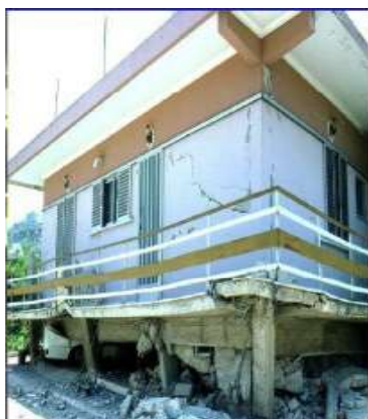
Fig. 3: Building damage due to effect of soft storey
